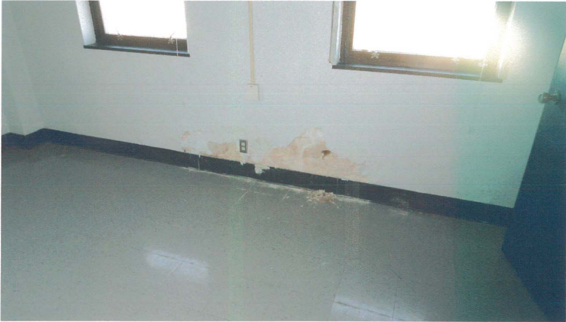
INTERIOR (water penetration damage)
