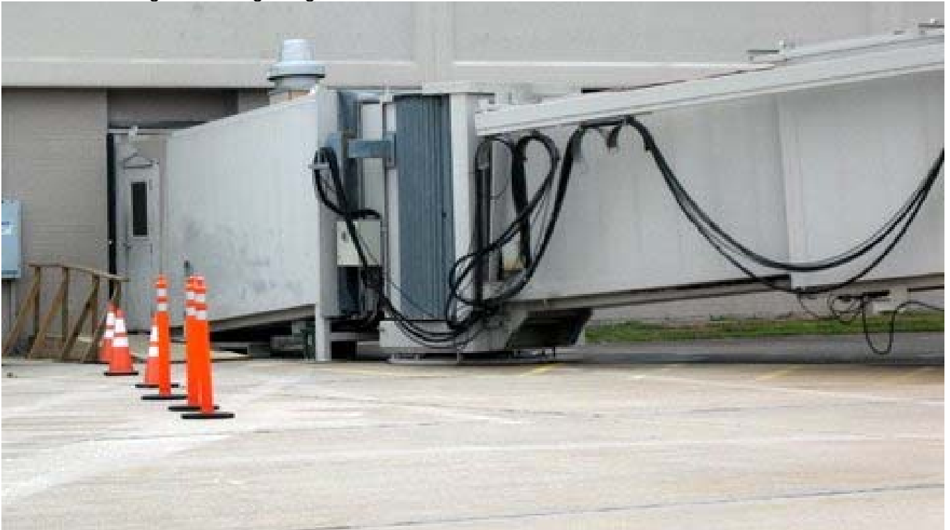
Photo of Passenger Boarding Bridge No. 2
