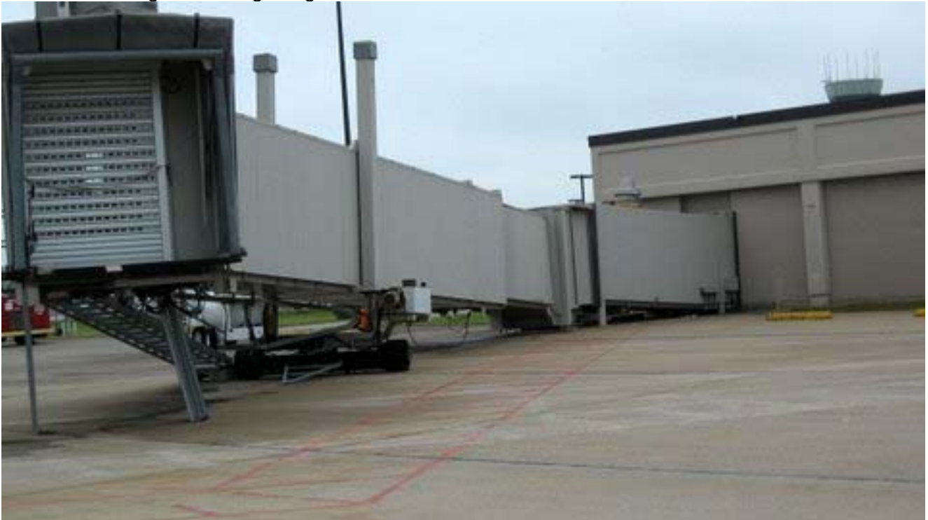
Photo of Passenger Boarding Bridge 1
