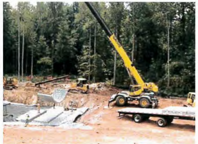
The use of a crane is optimal for fast and safe unloading and installation of the mats.
