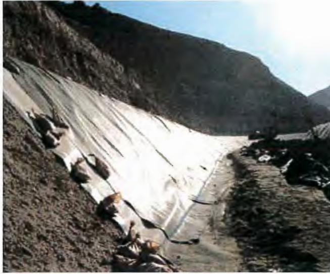
Fabric shall have the proper overlap and be free of any holes or tears.
