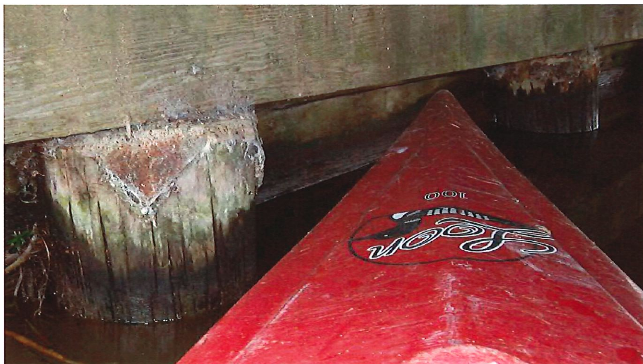
VIEW-32 NORTHEAST ABUTMENT PILES - LOOKING NORTHEAST JPEG No. : 0466 NOTE: INTERIOR TIMBER PILES AT NORTHEAST ABUTMENT HAVE ADVANCED DECAYED AT WATER LEVEL.
