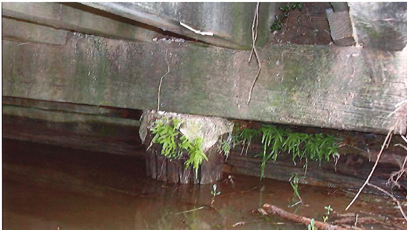
VIEW-31 NORTHEAST ABUTMENT SOUTHEAST PILE - LOOKING NORTHEAST JPEG No. : 0443 NOTE: SOUTHEAST EXTERIOR TIMBER PILE AT NORTHEAST ABUTMENT HAS ADVANCED DECAYED AT WATER LEVEL.
