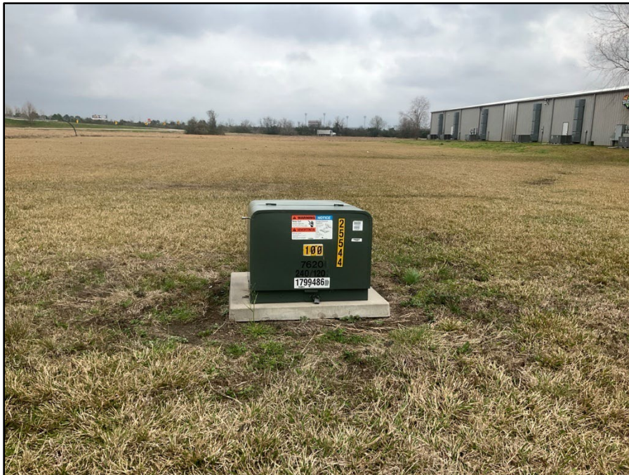
Figure 10. View of electrical box, facing northeast.
