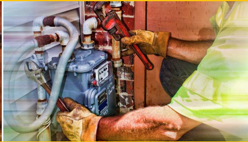
■ Gas repairs must be made by a licensed plumber and certified by city or parish inspector prior to restoring gas service.
